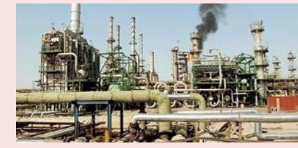
The Basrah Refinery was built in the 1970s by a Japanese company. Upgrade work will begin in the first half of next year, with the scheduled completion of 2025.
